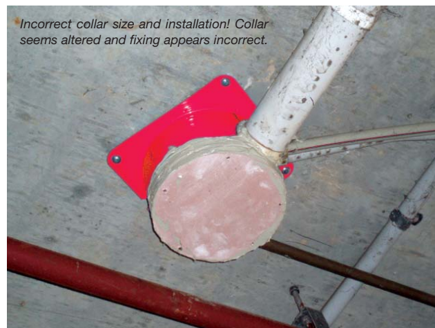
The retrofit collar is cut incorrectly. Pipe system also appears to be an untested system. Fixing also seems incorrect.
