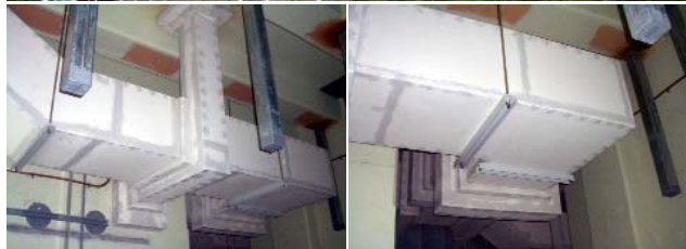
Ling'ao Nuclear Power Plant is located on the Dapeng Peninsula in the Longgang District of Shenzhen, Guangdong province, about 60km north of Hong Kong. The generator plant currently has two nuclear reactors and employs PROMATECT®-L500 self supporting ducts (above) among other proactive fire protection systems.
