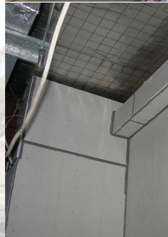
Above: Upgrade of 1 hour brickwork wall complete using 12mm PROMATECT®-H fixed to one side only. The structural steelwork above the wall is protected with 20mm PROMATECT® 250.
