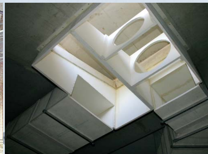
Above: PROMATECT®-LS self-supporting ductwork in Arena Düsseldorf, Germany.
