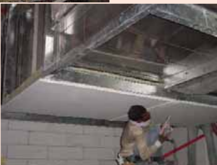
(Above) Specialist installer training conducted by Promat Singapore for installing the ducts in Changi Water Reclamation Plant.
