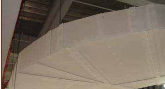
(Above and right) PROMATECT® -H smoke extraction ductwork in One Raffles Quay, Singapore.
