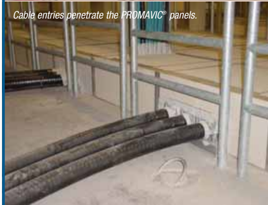
PROMAVIC® panels cover over cable ramp.
