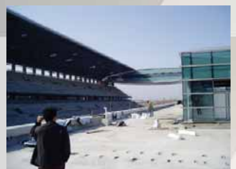
Top to bottom: The red towers – symbolic "guards of the entrance/gate" of the grandstand of Shanghai's new F1 circuit – feature PROMATECT® partitions in compartments around the towers.
