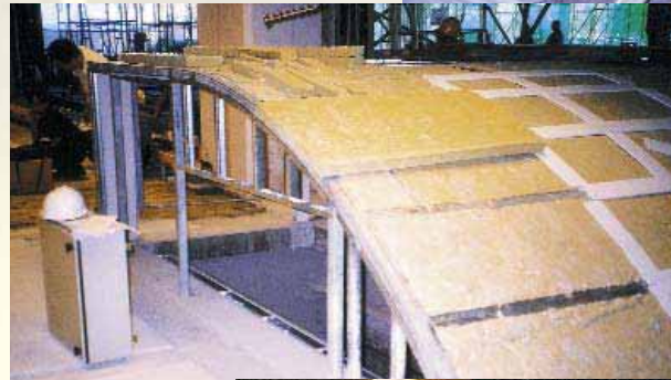
Building up the construction: First layer of PROMATECT®-H board beneath, followed by rockwool and cover strips.
