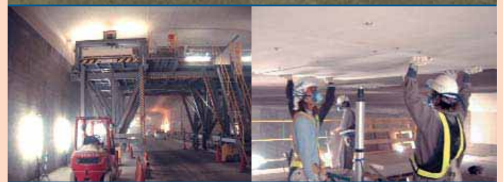
Above: Cladding construction method using PROMATECT®-H boards in Tokyo Port Seaside Road Tunnel.
