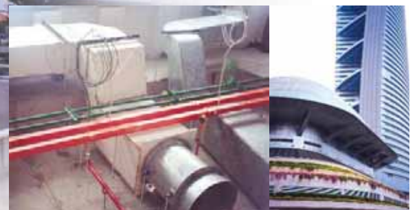
Right: Smoke extraction ducts play an essential role of safety protection in this modern architecture design building
