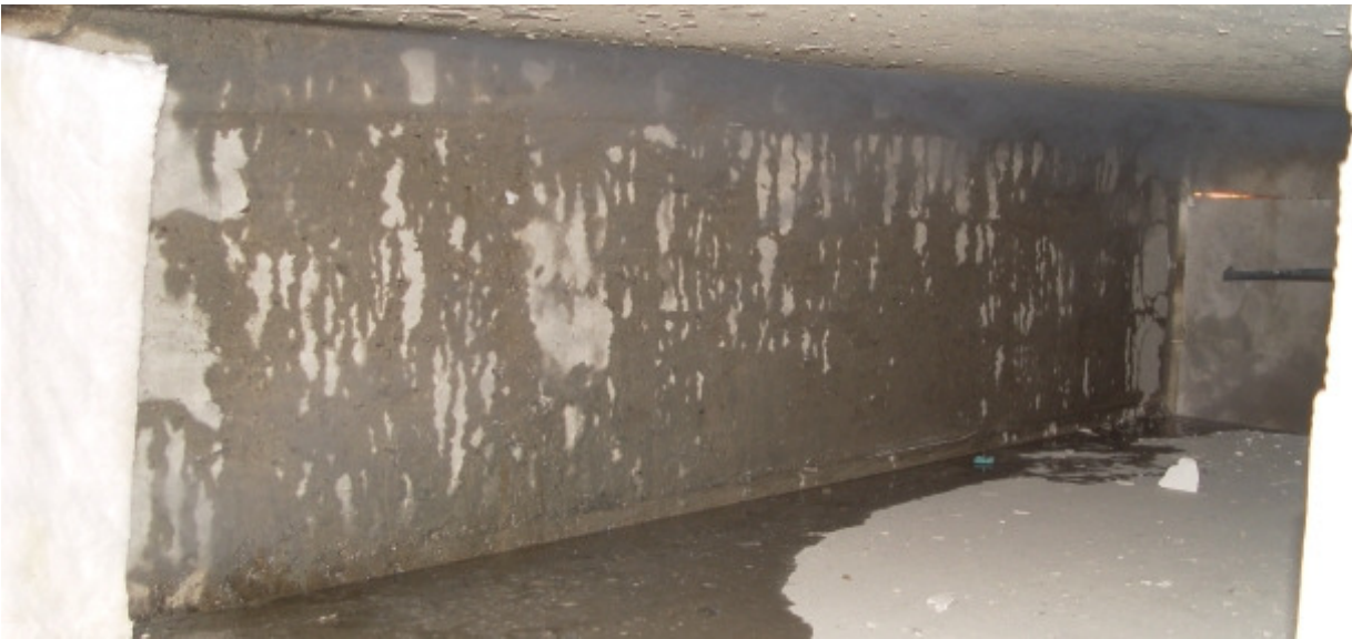
Water emerging from the middle wall after 30 minutes of heating. The photograph is taken from the unheated tunnel tube.
