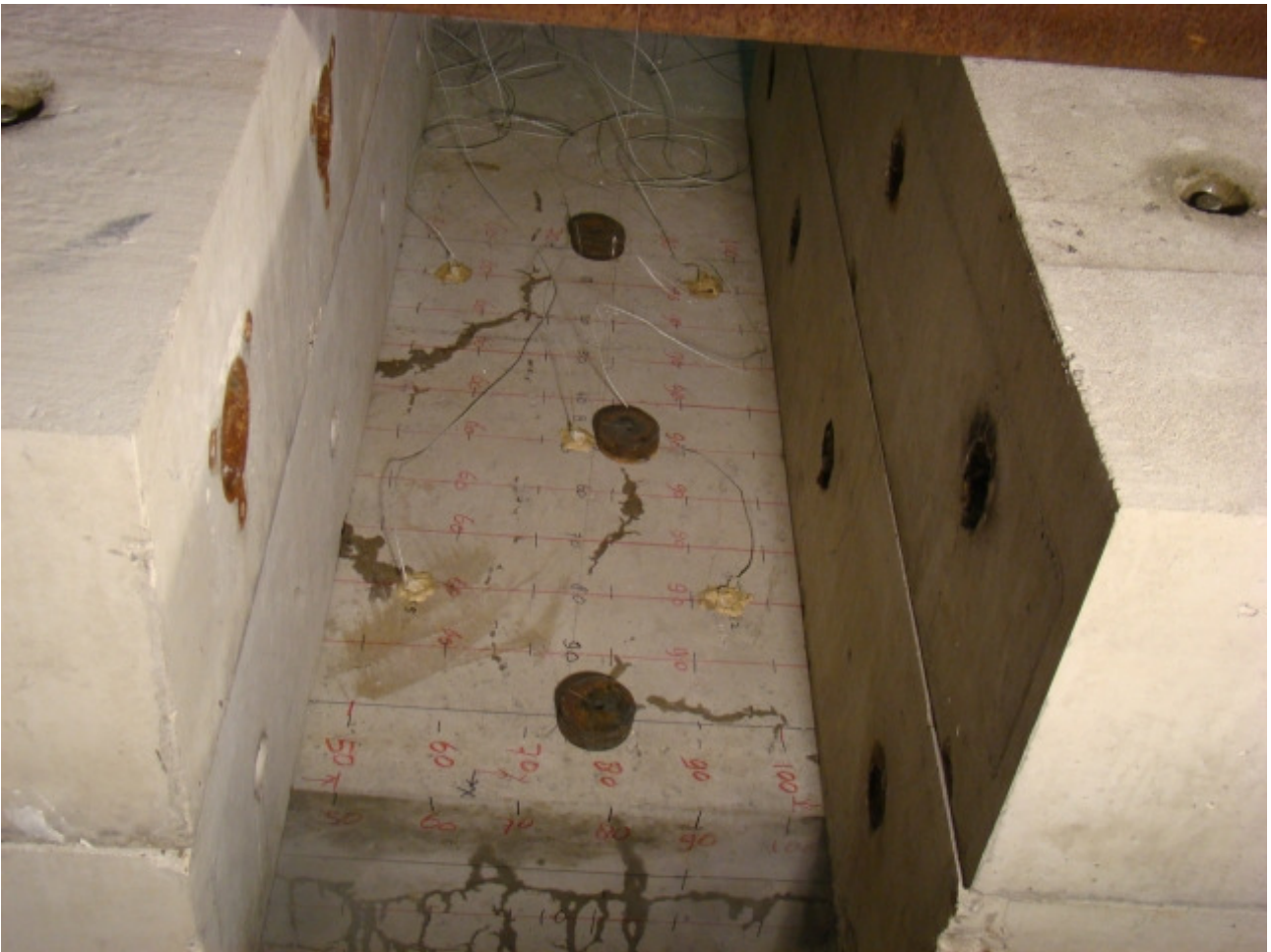
Only the small surface area between the blocks remained free for assessing crack widths.
